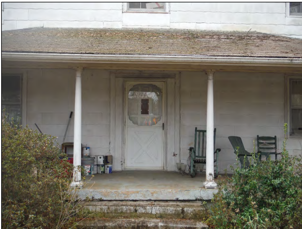
Figure 2.7.3. Detail of porch and entryway of the Houser House, residence, facing south.
