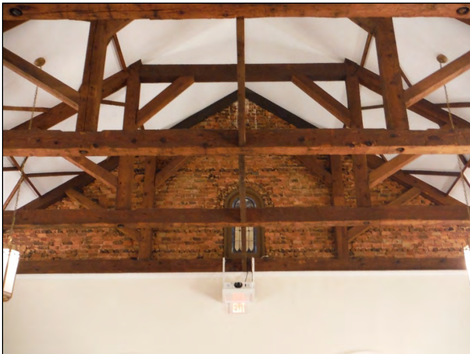
Figure 2.6.12. Interior of Gilead ARP Church, original structure, roof framing detail, facing northwest.
